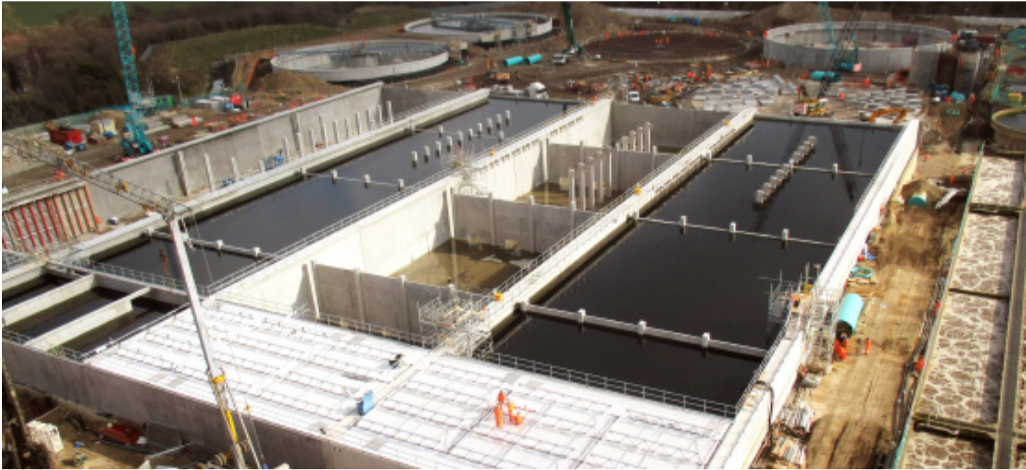
Deephams sewage treatment works
